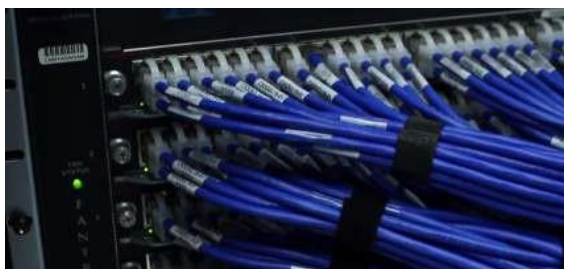
Source: HenryNewman12, CC BY-SA 4.0, via Wikimedia Commons [Internet cables plugged into a server]
